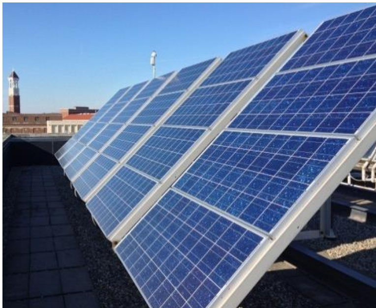
24-Panel Array with Weather Station
